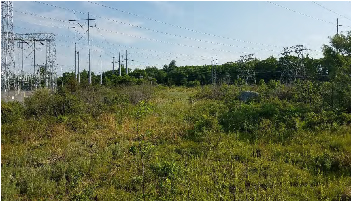
Photo #3: View of the K137/L138/337 Lines ROW near Sandy Pond Substation in Ayer, MA. Facing north east.
