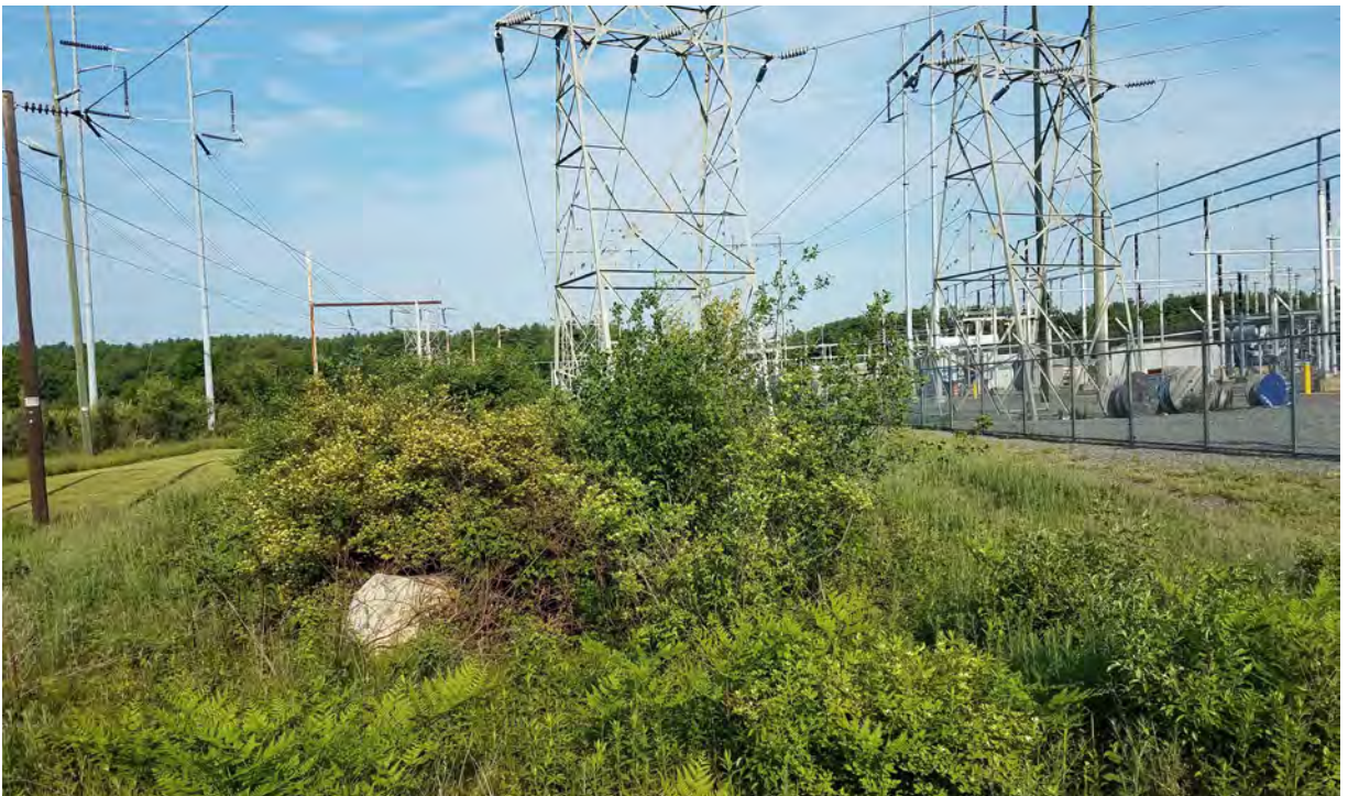
Photo #4: View of the K137/L138/337 Lines ROW near Sandy Pond Substation in Ayer, MA. Facing south west.
