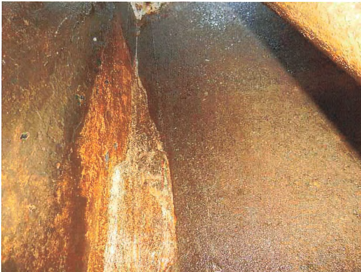
Photo 2: Crack with efflorescence (white staining) at lower portion of wet well walls.
