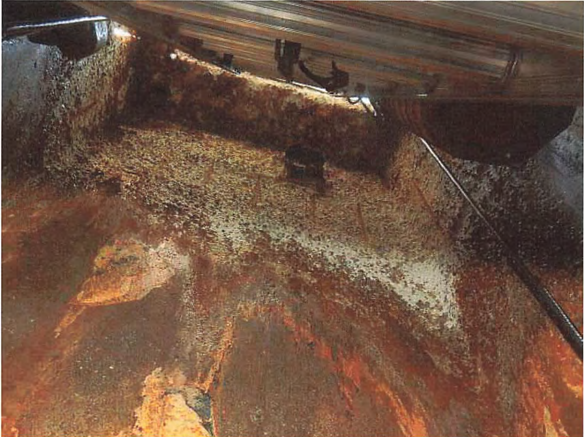
Photo 1: View of the upper portion of the wet well (primarily the north wall) showing loss of concrete cover and exposure of vertical reinforcement. Loss of concrete cover is also visible on the underside of the top slab.
