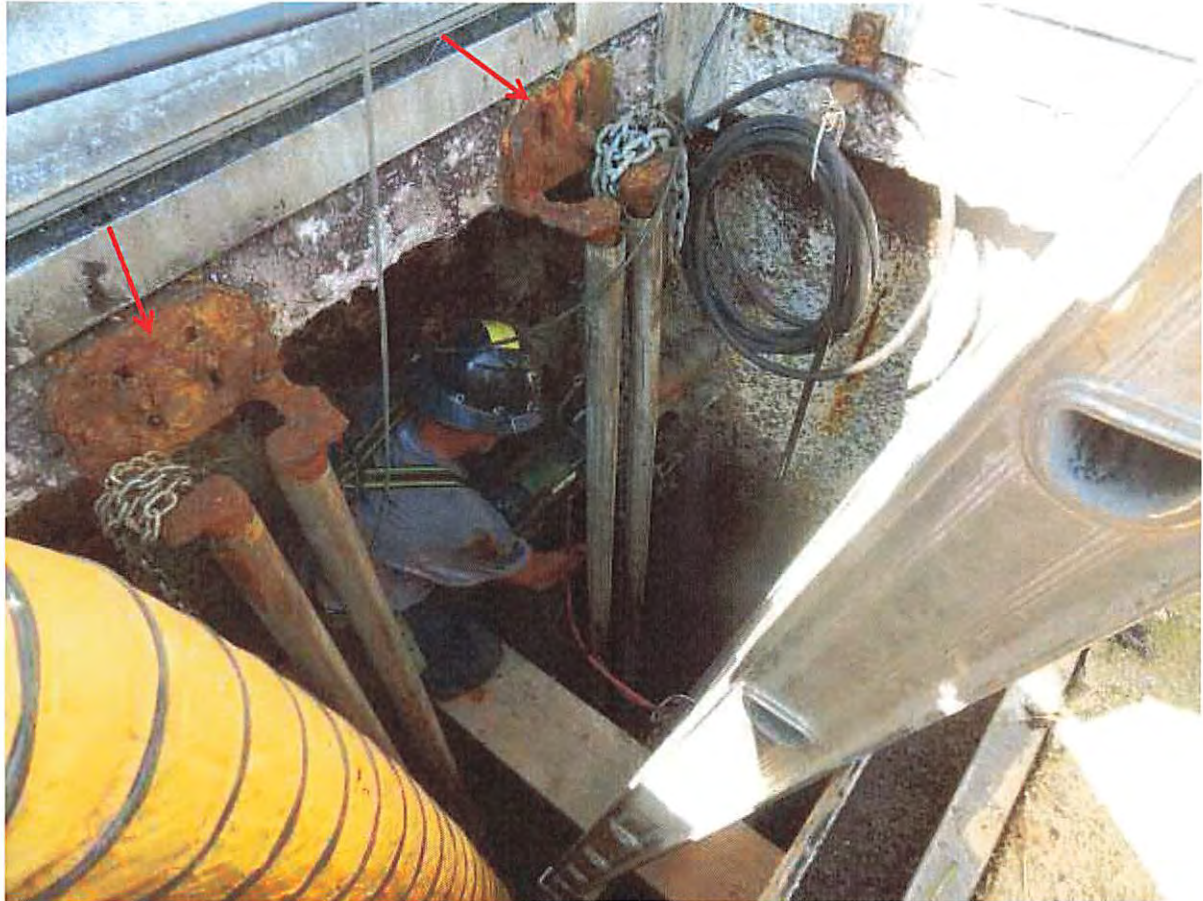
Photo 4: View of hatch opening during the coring operation for Core C-2 taken from the west wall. Note the severely deteriorated pump guide rail supports (red arrows).
