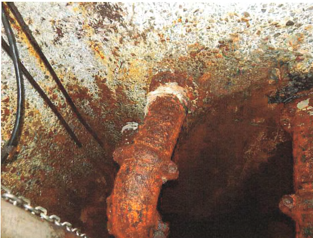
Photo 3: View of severely corroded piping within the wet well.
