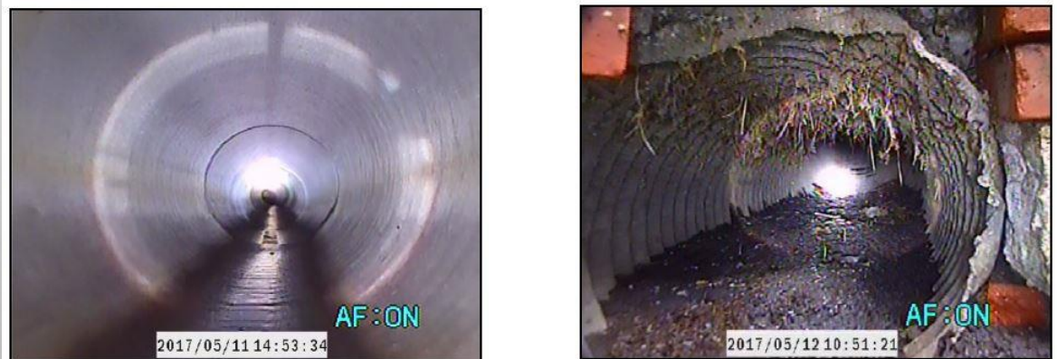
Figure 3-7 Example of a RCP in Excellent Condition (Left) and CMP in Poor Condition (Right)
