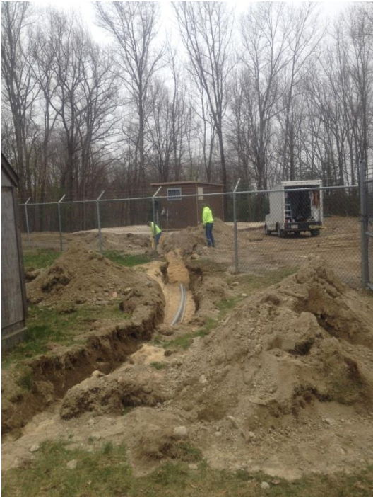
Power line run from wooden shed to concrete communications shelter
